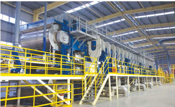
Difenbach continuous flat press (OSB board with thickness of 6.5mm~40mm, width of 2.5m and length of 12m can be produced)
